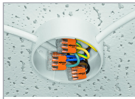
Lighting distribution in a ceiling canopy
