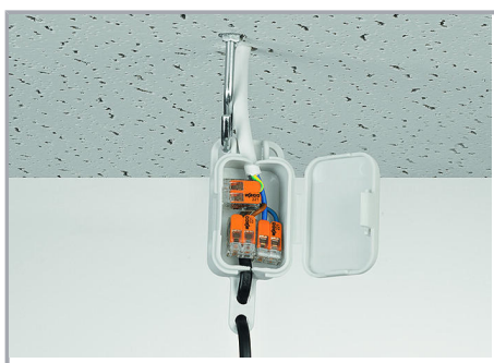
Pendant light connection in a suspended ceiling
